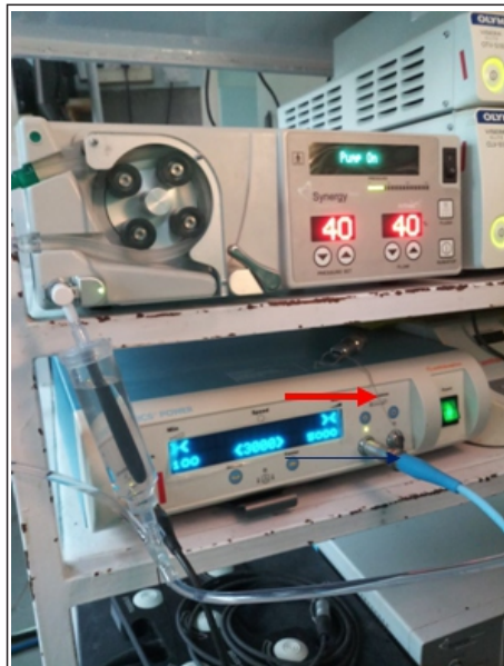
Figure 1: Irrigation pump with faulty sensor. The fluid level in the sensor is above the normal level.
